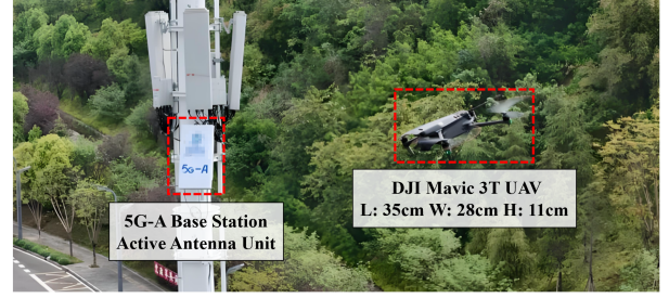
Figure 10: The 5G-A base station Active Antenna Unit (AAU) and the UAV deployed in our field experiments.
